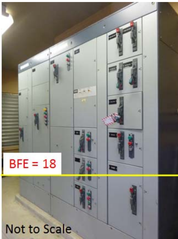
Figure 17 Smith Master Control Panel (MCC)
