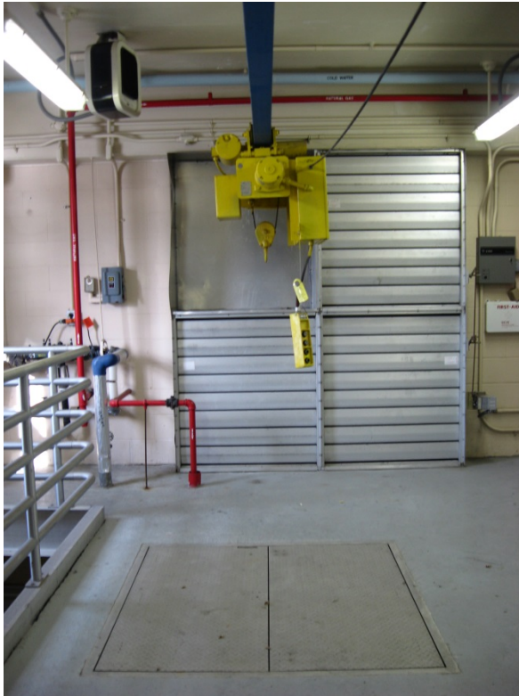
Figure 20 Louvered Opening for Equipment Removal
