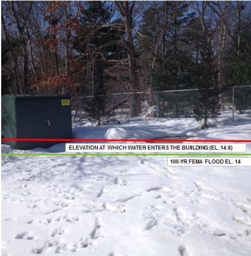
Figure 67 Linwood Pump Station
