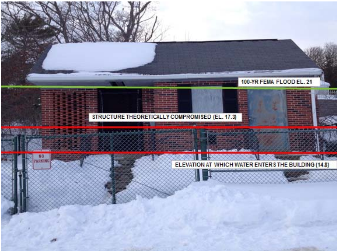
Figure 14 Saltworks Road Pump Station
