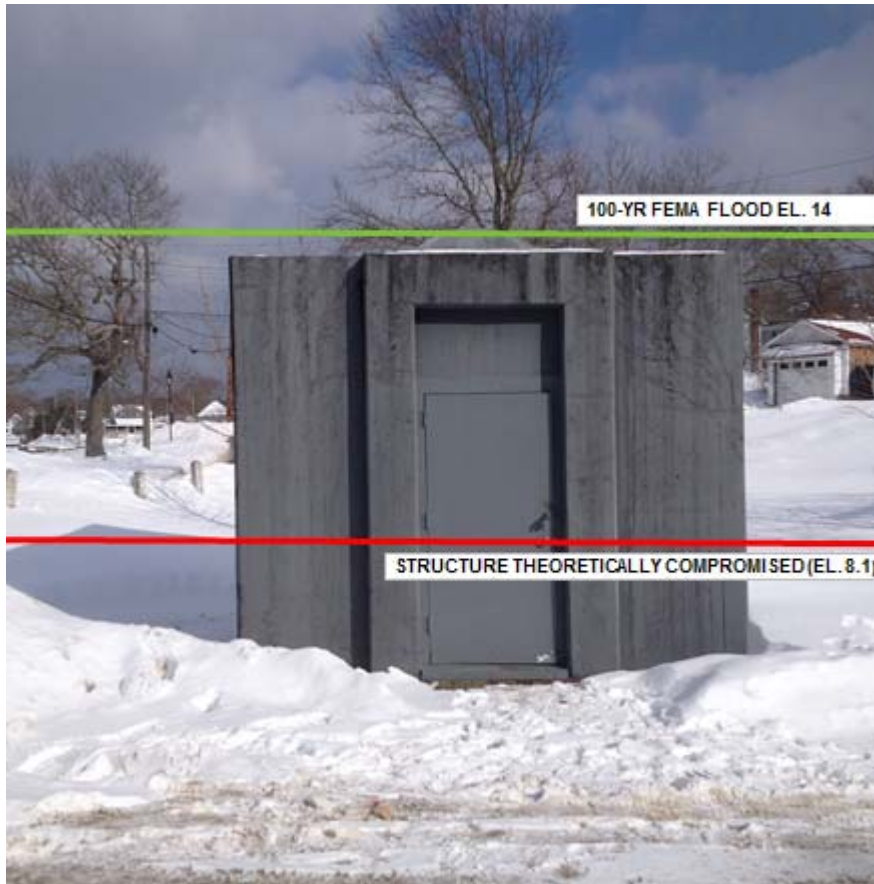
Figure 60 East Boulevard Pump Station
