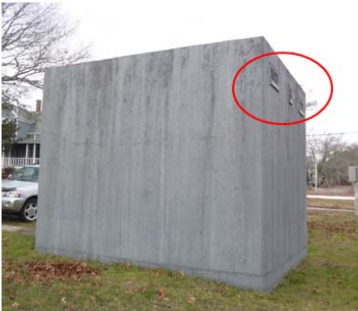
Figure 62 Water Entry Point at Vents
