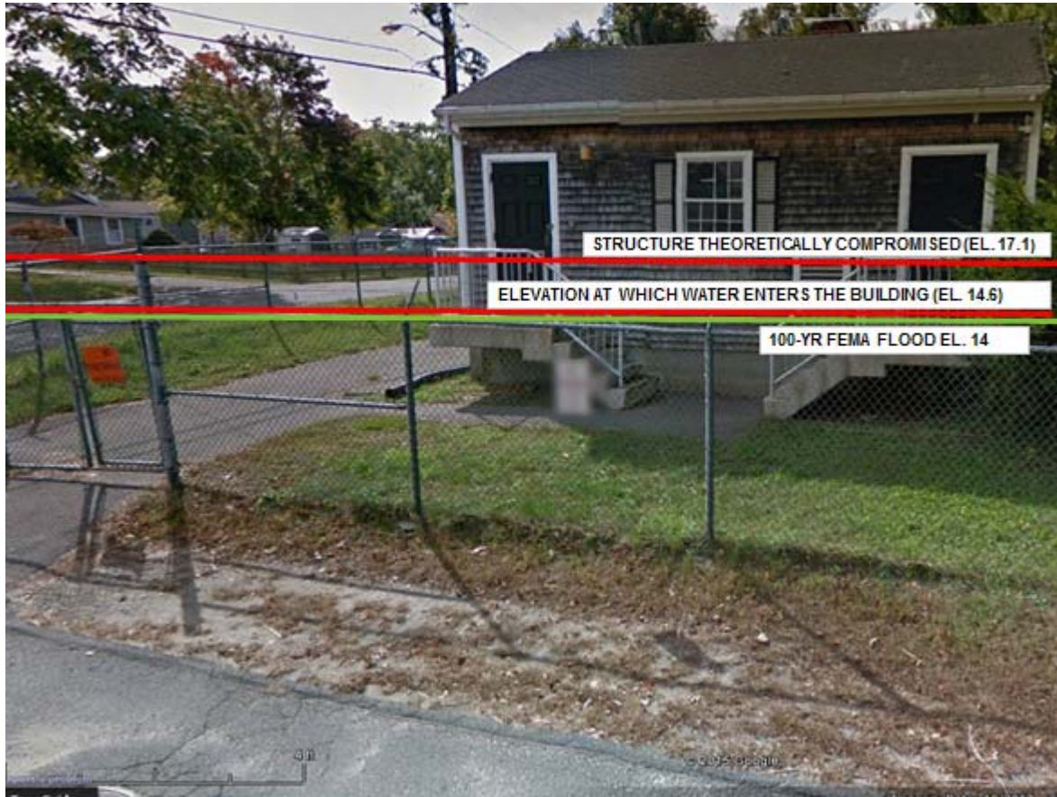
Figure 48 Pinehurst Pump Station
