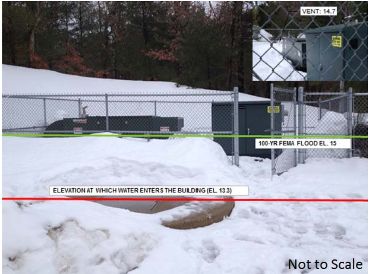
Figure 63 Parkwood Pump Station
