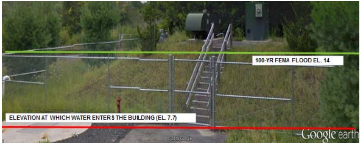
Figure 65 Indian Neck Pump Station
