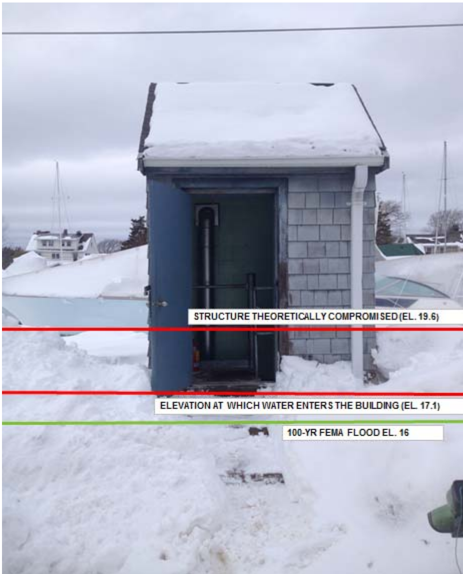
Figure 73 Green Street Pump Station
