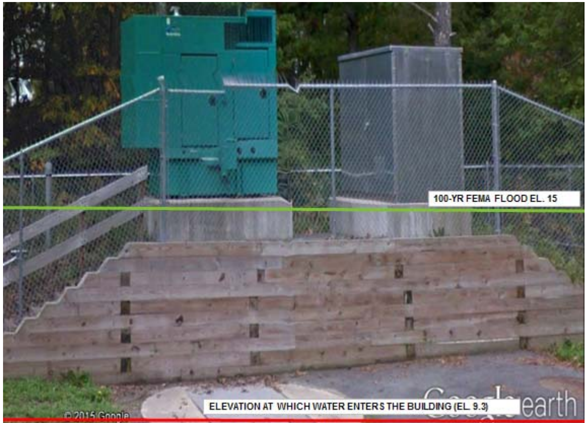
Figure 41 Briarwood Pump Station
