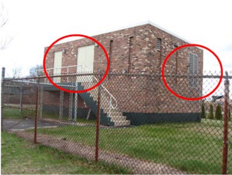
Figure 58 Potential Water Entry Points: Doors and Louver
