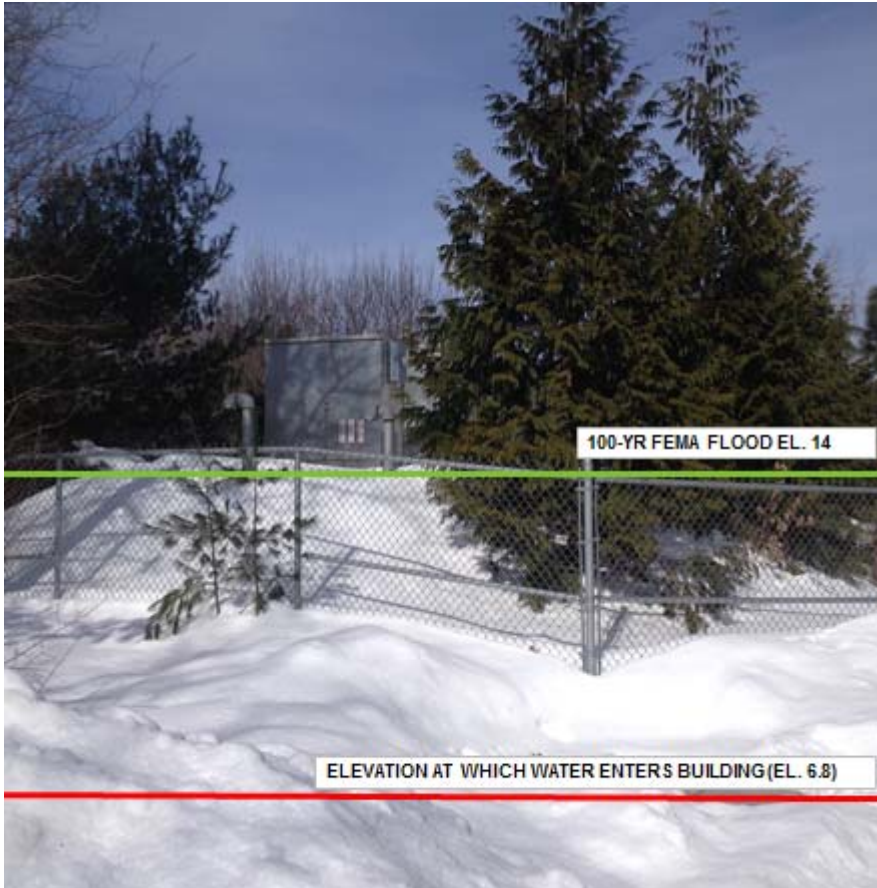
Figure 43 Arnold Pump Station
