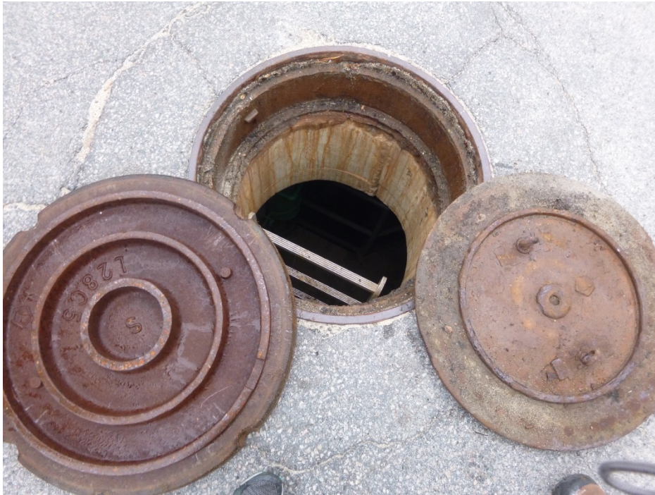
Figure 7 Bay Street Watertight Manhole Cover
