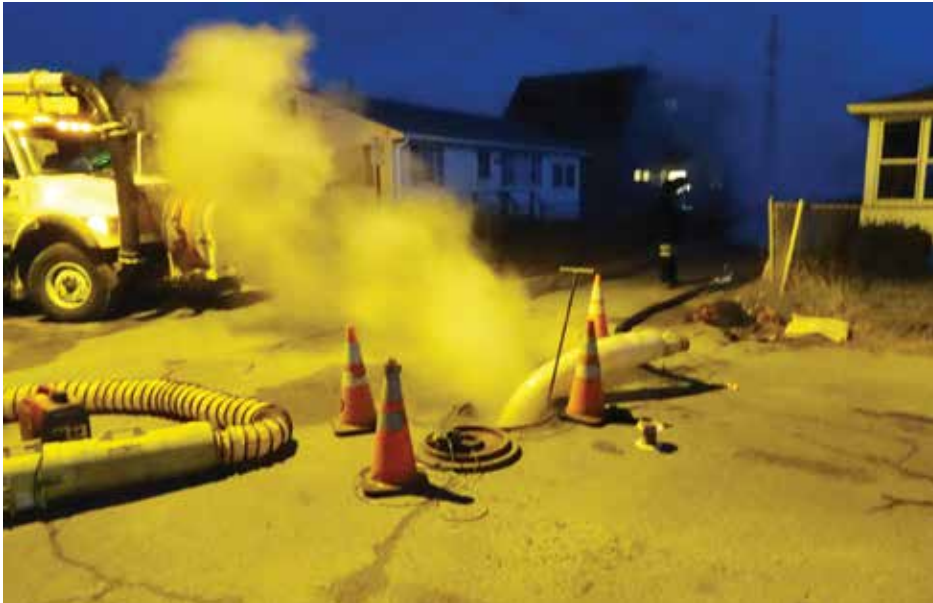
Lining & curing pipe into the night. The neighbors could not have been more hospitable
