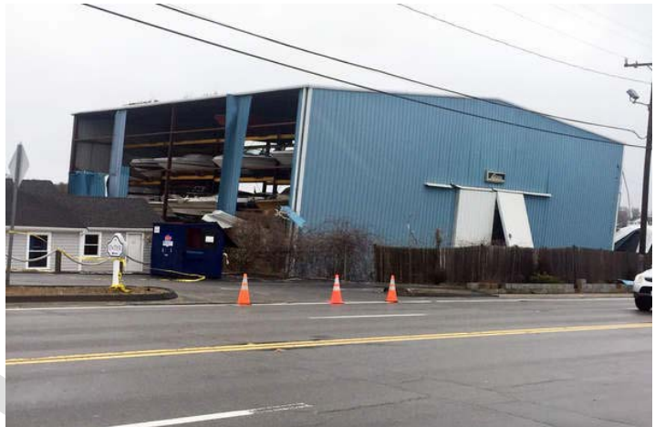
Figure 4: Boat storage facility on Cranberry Highway suffered irreparable damage from the March 2018 Storms.
