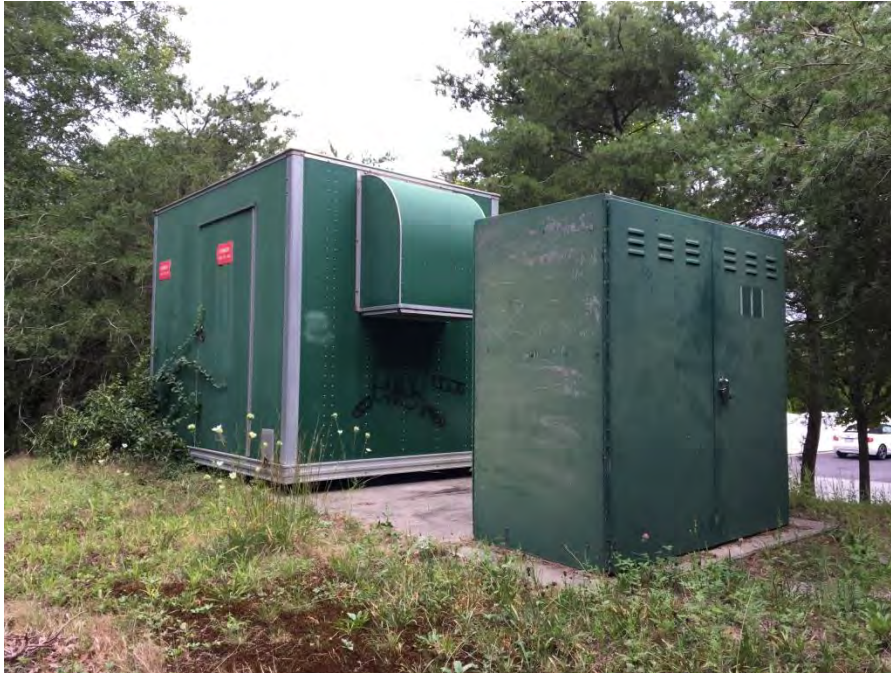
Figure 4-5. Onset Heights Pump Station.
