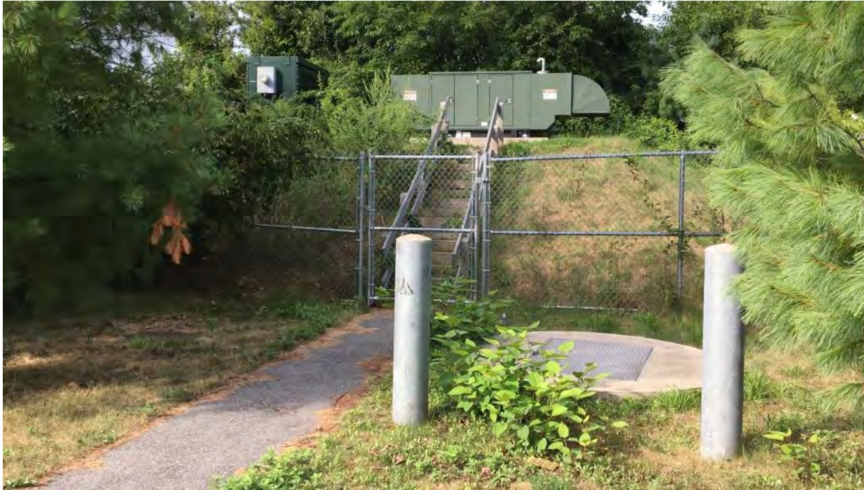
Figure 4-9. Avenue A Pump Station.
