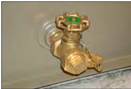
Figure 3. Drain valve with sampler.
