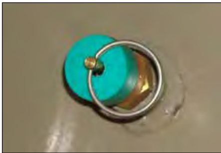
Figure 4. Automatic Pressure relief valve.
