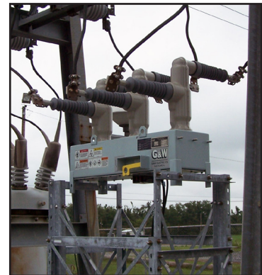
▲ Custom mounted frame required for replacement of previously installed oil filled equipment.
