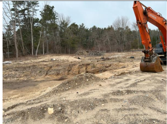
Photograph 2 – In progress Stormwater basin with erosion
