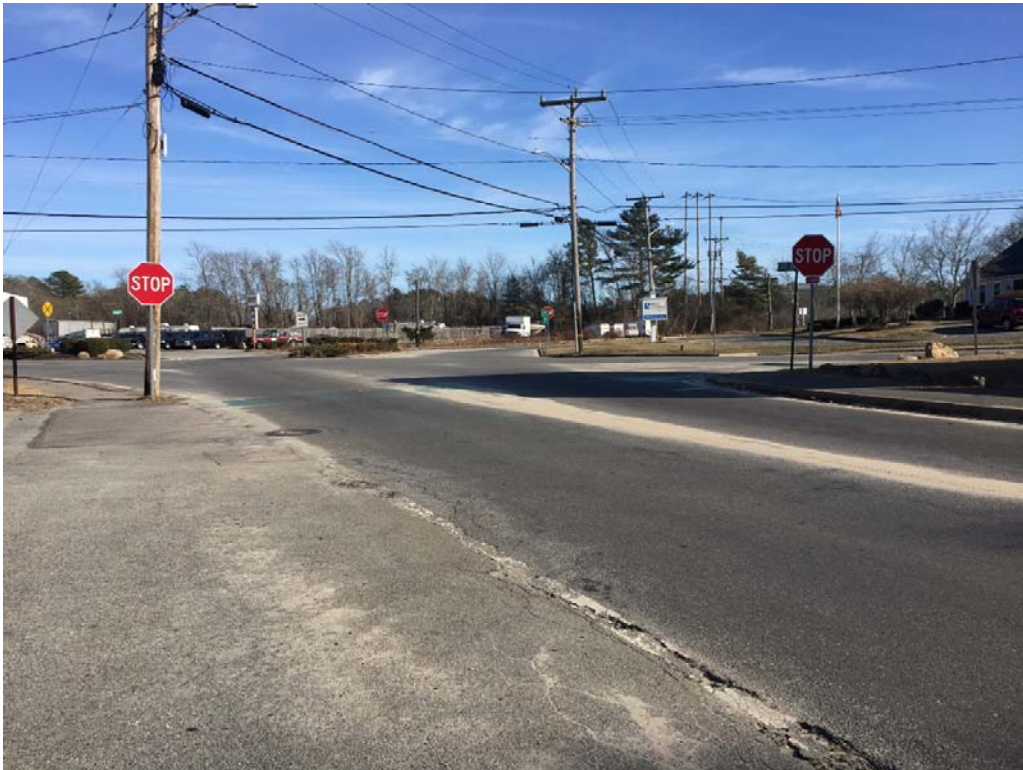
View of intersection at Minot Ave and Depot St looking Eastbound at STA point 93+00 +/-
