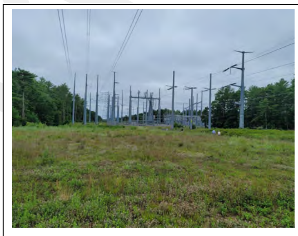
Figure 7 – North of Site – View to the West of Eversource Substation (view as of 13/Jul/2021)
