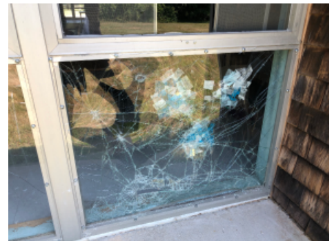
Vandalized glass in the E wing.
