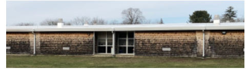
Cedar shingles have been replaced throughout the building including areas next to the new downspouts
