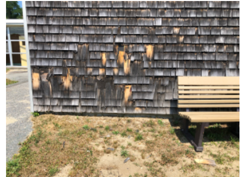
It appears damaged shingles are being pulled off the building near the playground.
