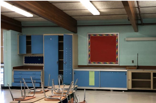
Typical classroom unit ventilator is concealed in the blue cabinet on the right.
