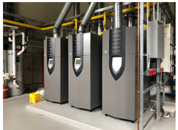
Three new boilers installed in 2017. New hot water heaters in background.
