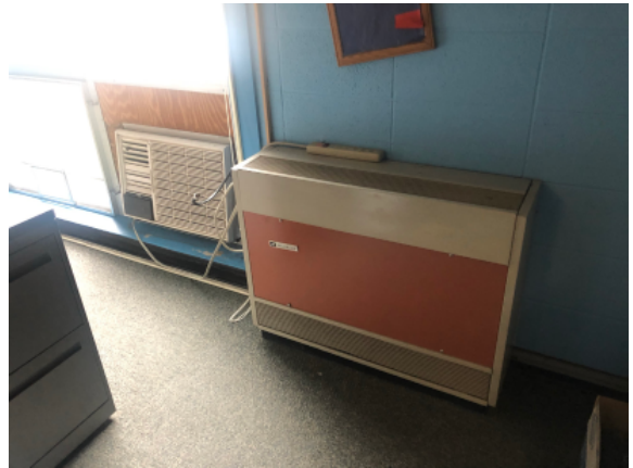
Typical non-classroom unit ventilator and air conditioning unit.
