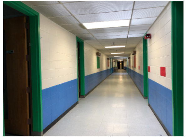
B Wing hallway, a typical hallway layout throughout the building. Above each cluster of four classroom doors there are plastic mesh panels inset in the suspended ceiling which allow sunlight to come in from skylights in the roof.
