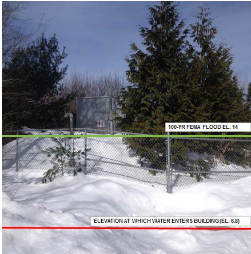
Figure 43 Arnold Pump Station
