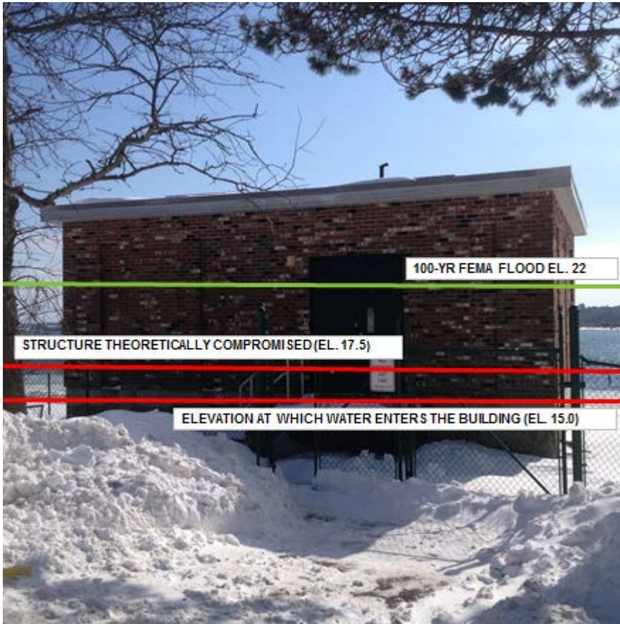
Figure 25 Onset Pier Pump Station
