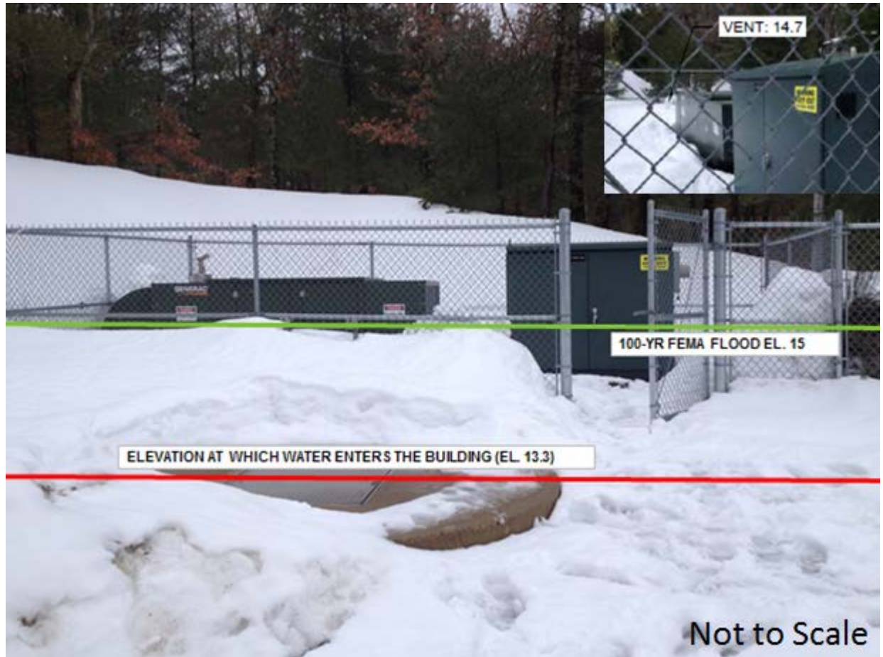
Figure 63 Parkwood Pump Station
