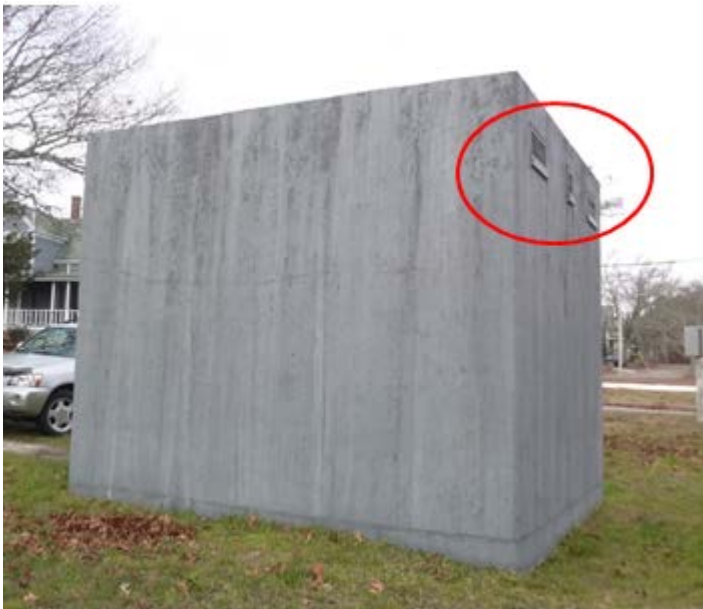
Figure 62 Water Entry Point at Vents
