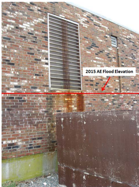
Figure 46 Narrows Pump Station Potential Water Entry Point
