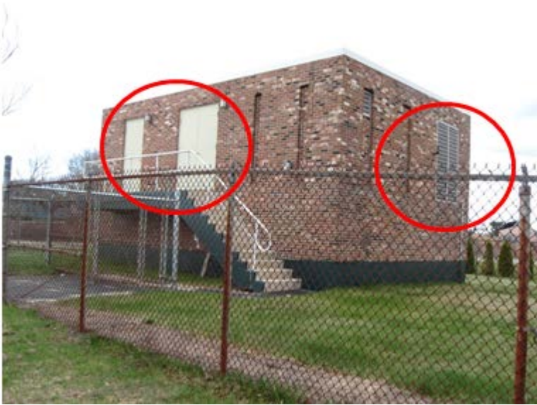
Figure 58 Potential Water Entry Points: Doors and Louver
