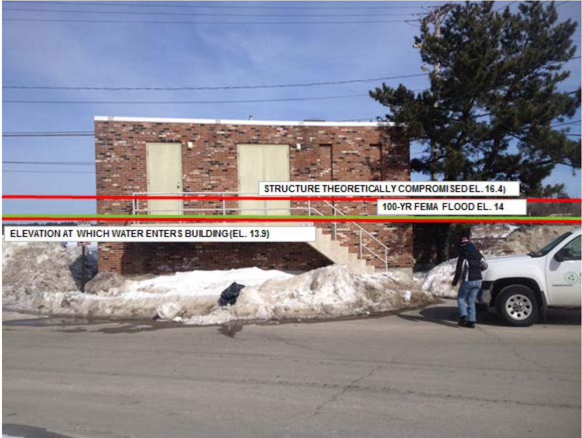
Figure 45 Narrows Pump Station
