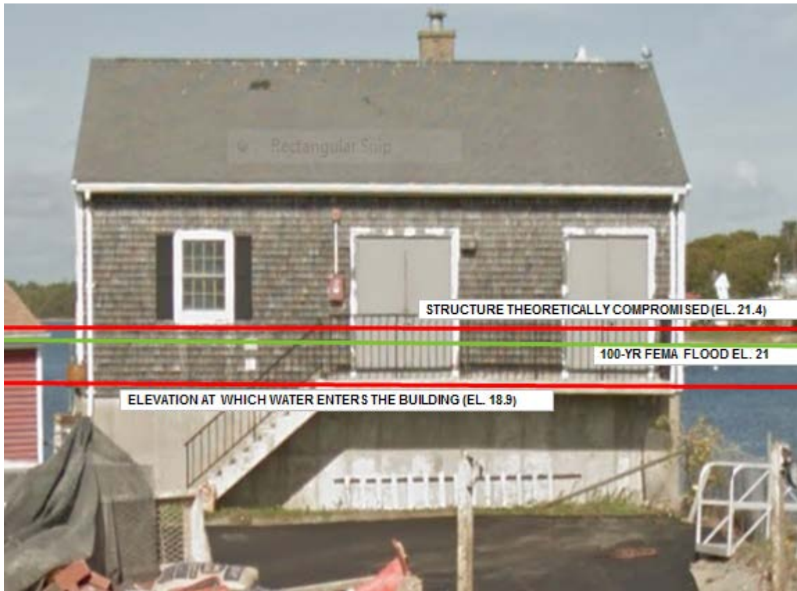
Figure 19 Cohasset Narrows Pump Station
