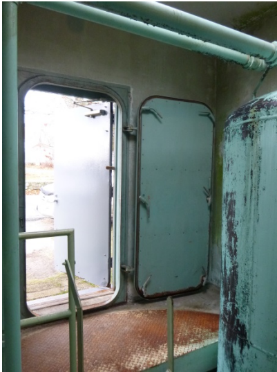
Figure 61 East Boulevard Watertight Door
