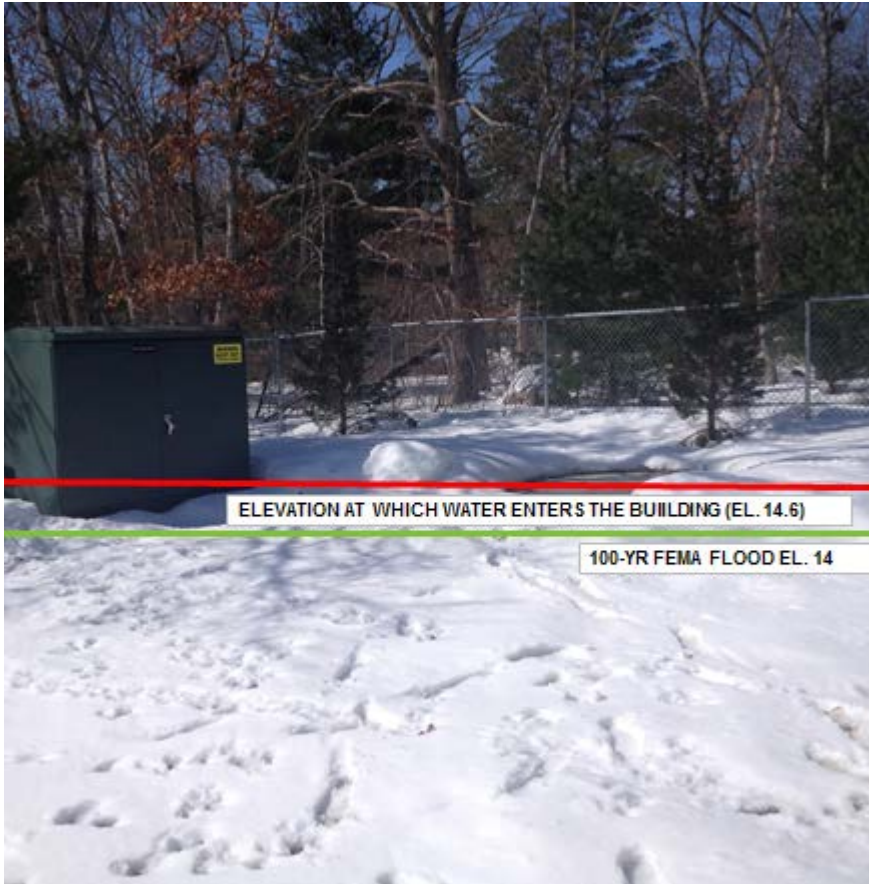
Figure 67 Linwood Pump Station
