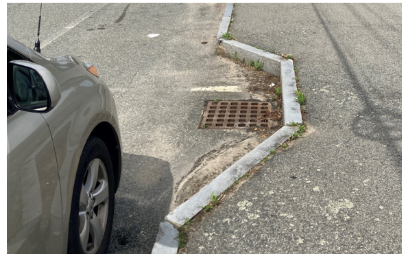
Untreated Stormwater Runoff
