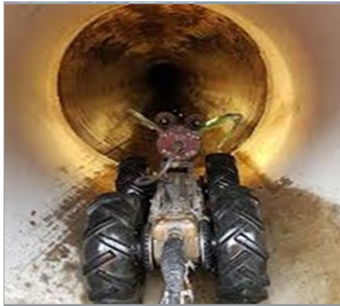
Illustration 11: CCTV crawler inside the host pipe
