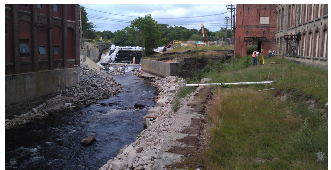
Pre-Construction Condition - Failure of river walls due to the 2010 flood.
