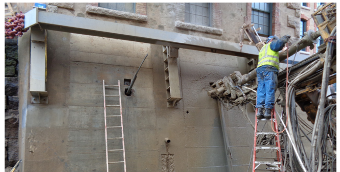
Installation of drilled tie-back anchors - To minimize the risk of further damage during construction, the Anthony Mill Tower was stabilized with an innovative system of concrete collar walls with micro-piles and drilled tie-back anchors.
