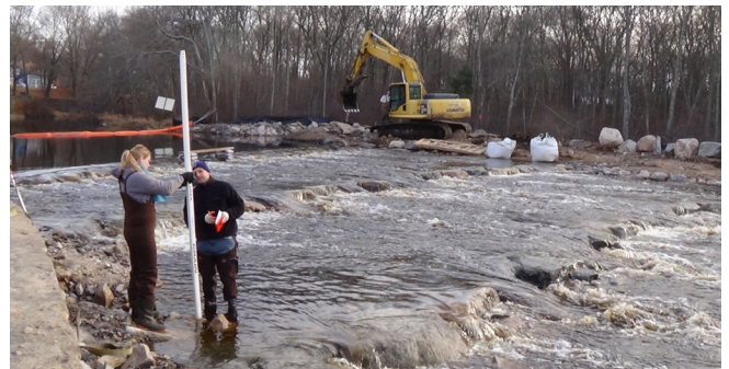
Field Investigation - Performed hydrologic/hydraulic analyses of flood flows and prepared FEMA floodplain map revision submittals; conducted field investigation of impounded sediments; and developed design to minimize mobility and impacts to upstream bridge.
