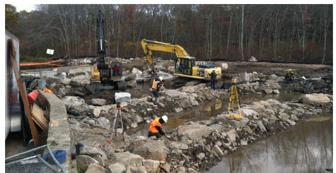
Fish Passage Construction - Developed construction phasing to ensure that headpond elevations were maintained for the mill's fire suppression system.
