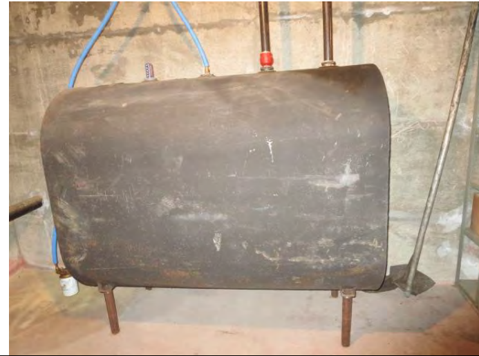
Photo #10: 275-gallon AST associated with the emergency generator.
