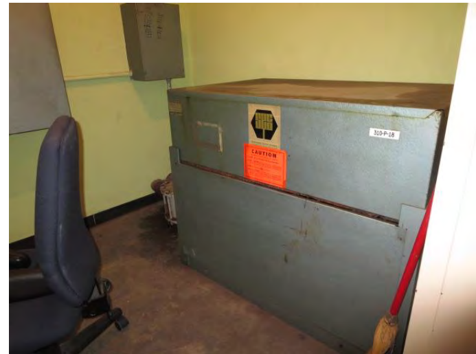
Photo #12: Hydraulic elevator equipment.
