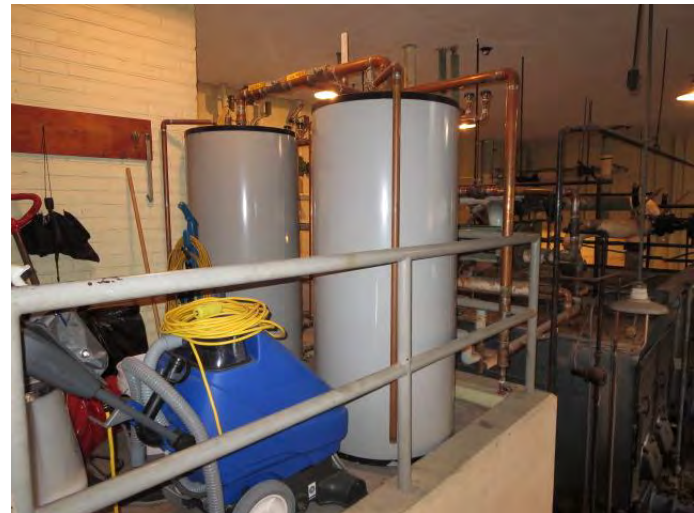
Photo #8: Water heaters.
