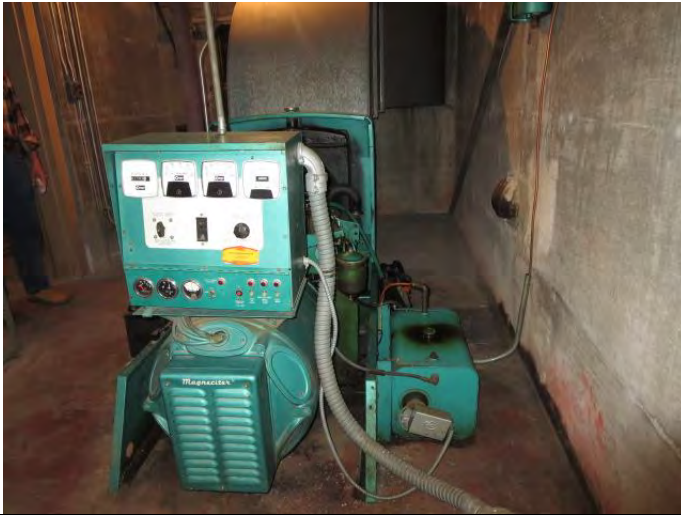
Photo #9: Emergency generator.
