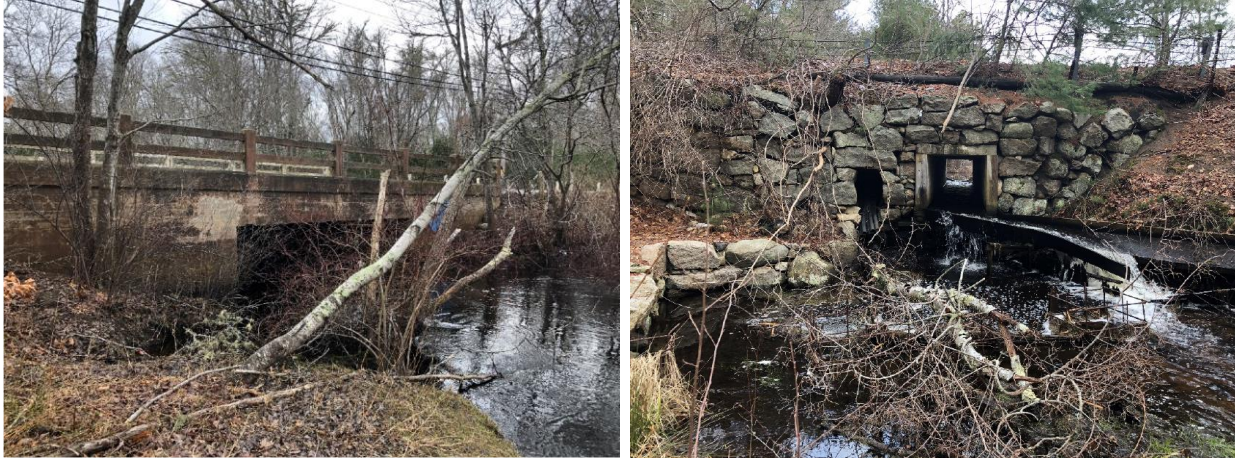
Figure 3-27. Fearing Hill Road Bridge (left) and Main Street culvert at Old Trout Farm (right).
