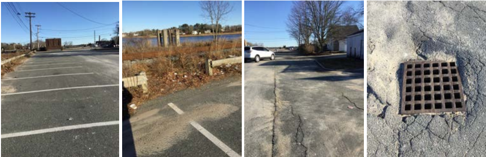
Looking southerly where pavements abut. This wide open area is unsafe and pedestrian unfriendly.
