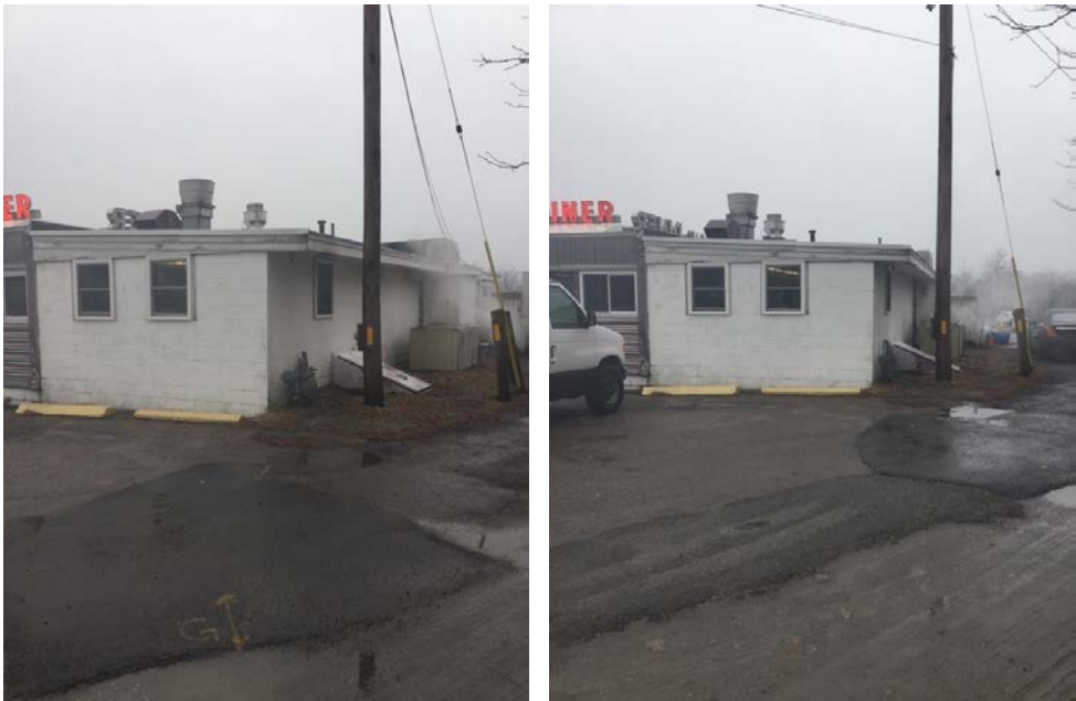
Rear of building; exterior walls in need of upkeep
