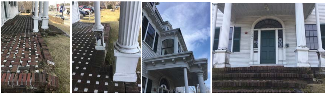
Details of Front Porch – Damaged trim, structural elements, and paving
