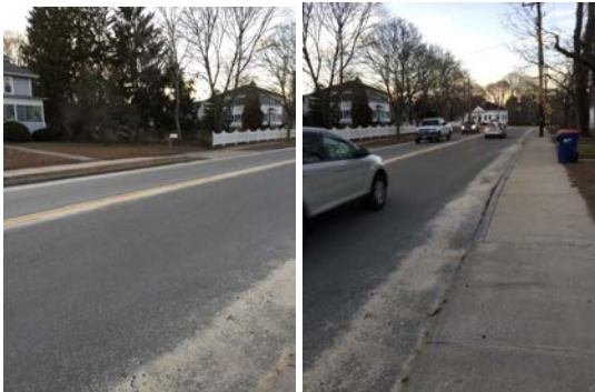
Looking northerly along easterly side of roadway. Everything in good shape except narrow sidewalk.
