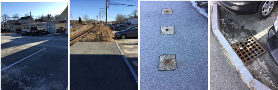
End of sidewalk with no hp access to pavement. Possible bench location within sidewalk, that has been removed.
