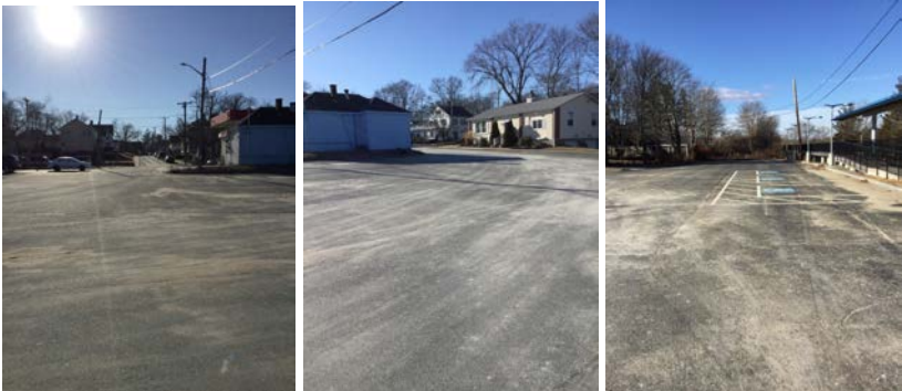
Parking area near RR platform. No islands and area is not pedestrian friendly.
