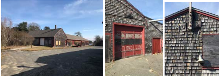
Siding deteriorating on main buildings
