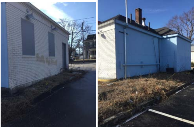
Graffiti and paint deterioration on the rear walls
