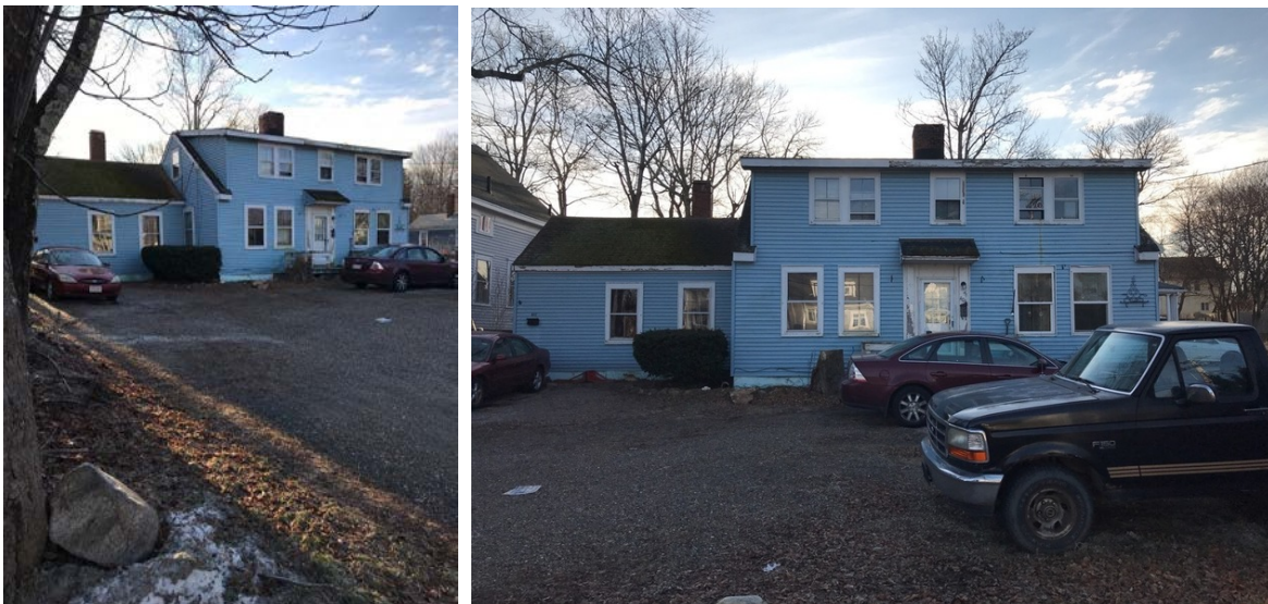
Exterior of house in poor condition, with rotted wood trim and entrance deteriorated
