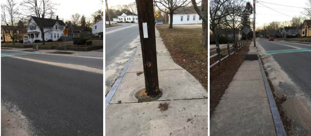
View looking southerly at westerly side of Main Street. Water line and hydrants can be found in grass strip.
