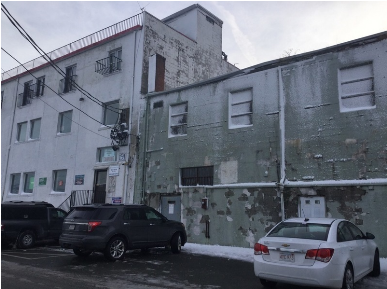
Rear of property with parking lot; faded white paint on back and right side
