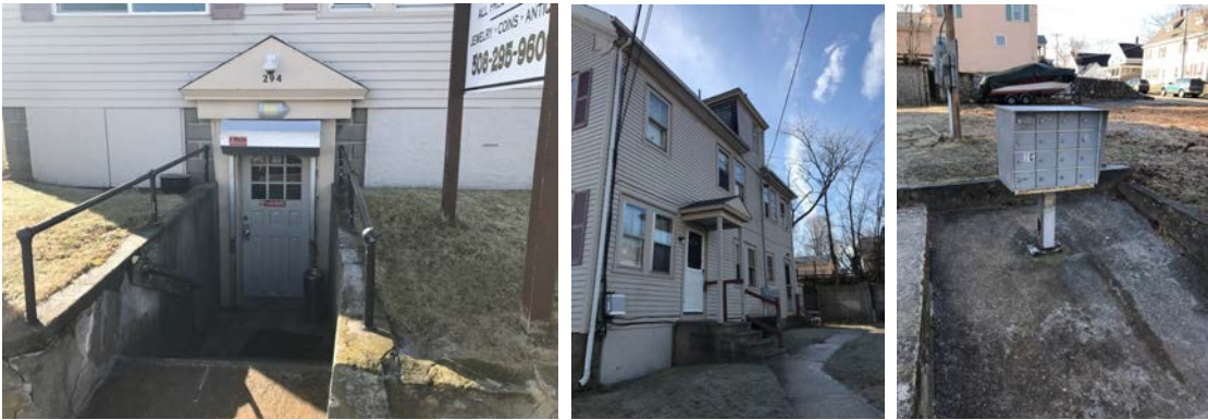
Entrances to building – five overall – entrance to store is poor and others are fair.
