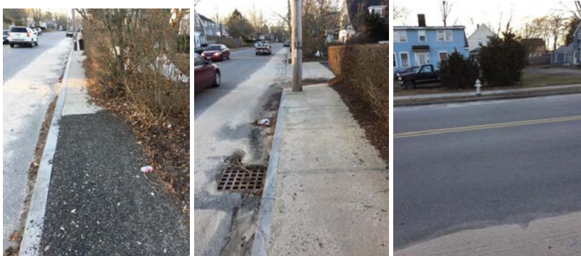
Another area where sidewalk was removed when telephone poles were replaced.
