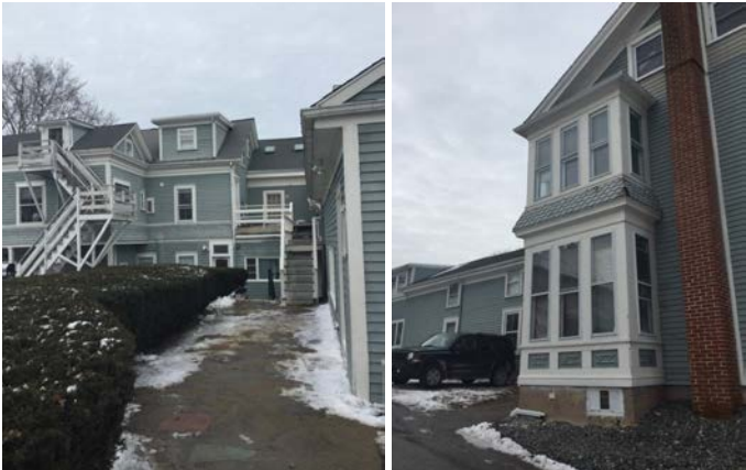
Rear side of main building; stairs and back porch in fair/poor condition
