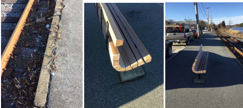
The railroad side of this area has an asphalt, sidewalk with benches (some vandalized).
