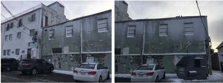
Rear of building and parking area; chipping paint on back wall and plant growth from edge of roof.
