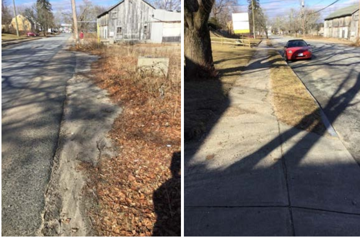
Impact of no curbing along side of Main Street.
