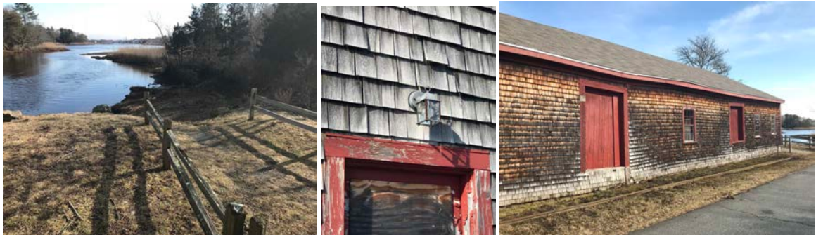
Property backs up to water; damage on exterior includes deterioration of siding, bees nest in lighting fixtures
