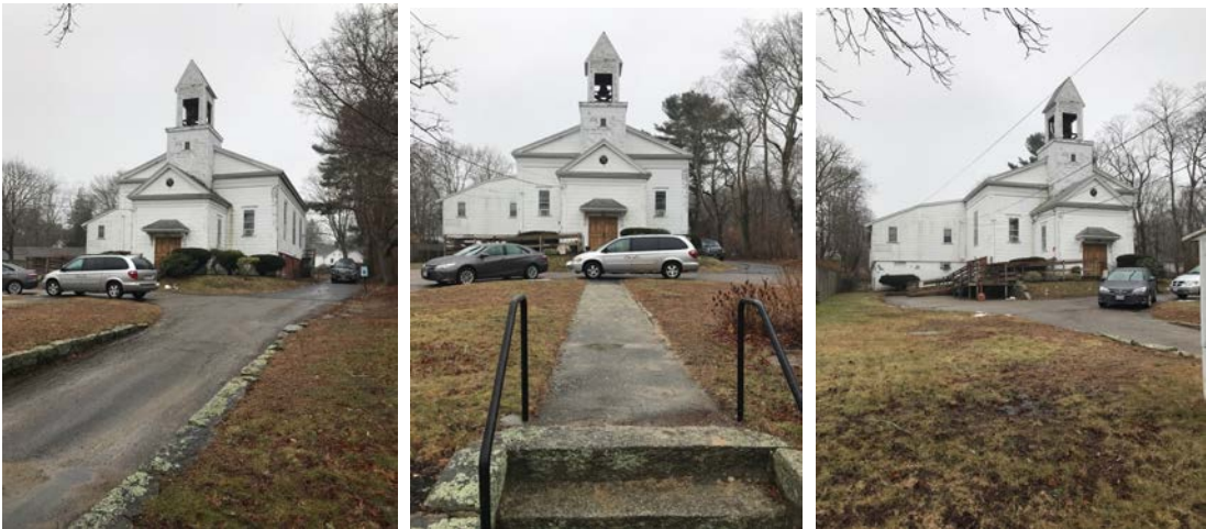
Building, with driveway and front pathway. Exterior siding in need of painting and repair.
