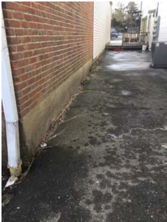
Side alley; roots growing from under foundation
