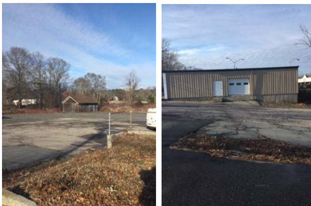
Two outbuildings: first a small shed in fair condition and second an aluminum sided vacant office type property in good condition.
