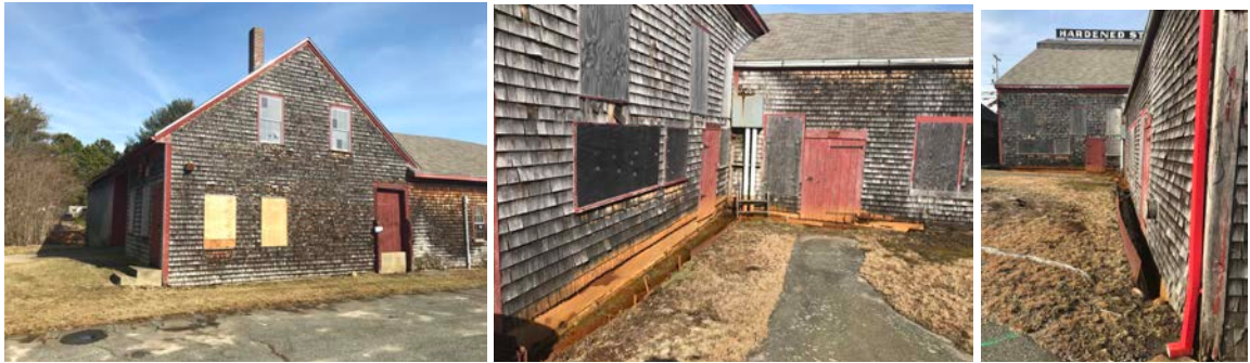
Windows and doors boarded up; paint on trim chipped
