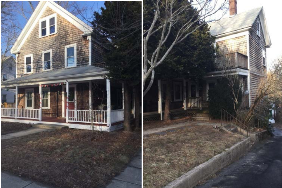
Front facing side of house with porch slightly crooked; right side of house
