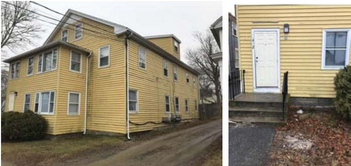
Rear of building, siding with discoloration; front door
