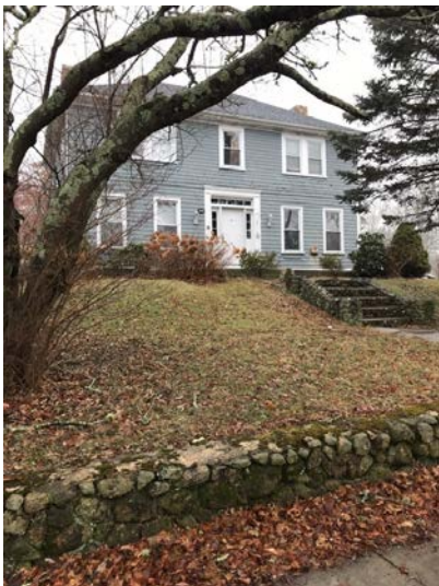
Some missing shingles and steps missing railings
