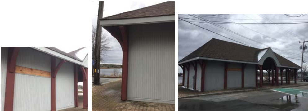
Exterior of the train station; one boarded up window
