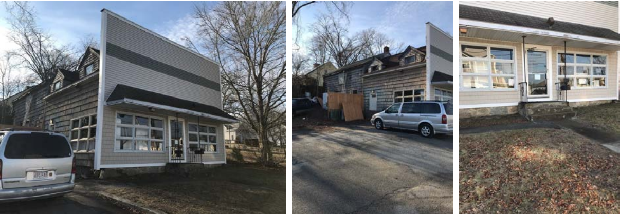
Front façade and side of structure; side roof badly deteriorated and several broken windows
