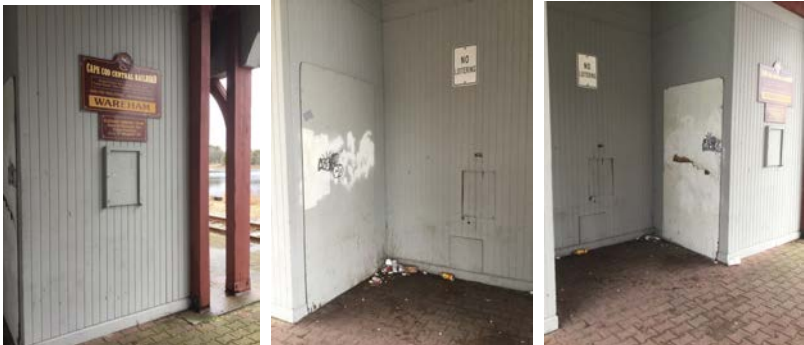
Inside of the train station; debris and graffiti on the boarded-up doors
