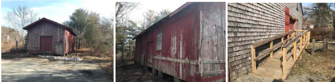
Rear structure paint deteriorating
